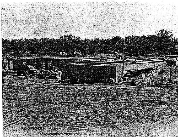
View of foundation of Provincial Offices and Residence, under construction on west side of Highway 31 and across from Dujarie property. Roof of building at right background is Dujarie Scholasticate, the Brothers' house of studies at Notre Dame.
