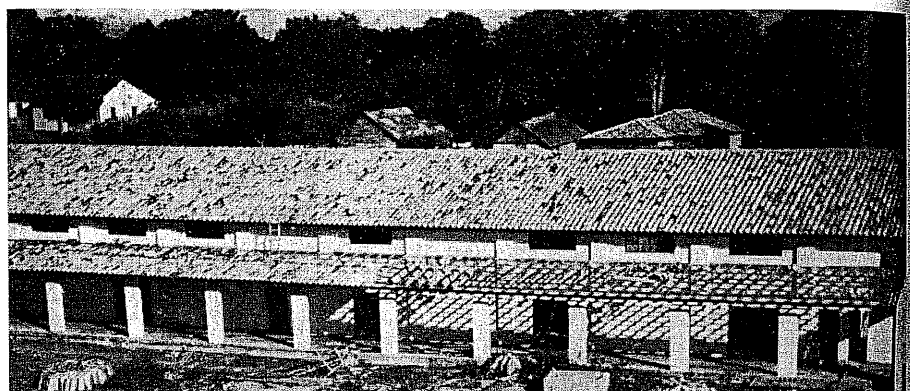
A new unit is almost completed for the Ginasio Dom Amando, Santarem, Para, Brazil.
