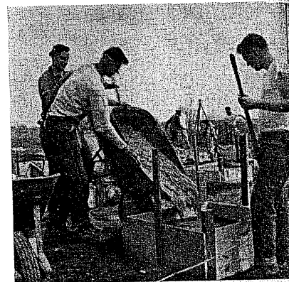
Left to right: Brothers Patrick McDonagh, Hugh Lennon, and Joseph Hogan pour concrete into one of the forms for foundation of the annex to Vincent Hall while others in the background tend the concrete mixer.
