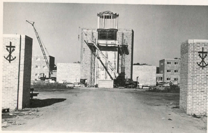
St. Joseph of Holy Cross Chapel—designed to serve the religious needs of the Holy Cross Junior College and for all major religious functions of the Midwest Province.
