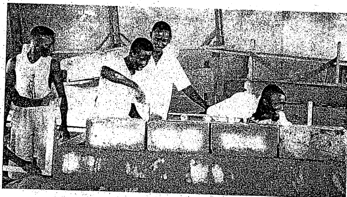
Br. Daniel Dardoe (second from right) supervising masonry training at the Holy Cross Skills Project, Sekondi, Ghana.
